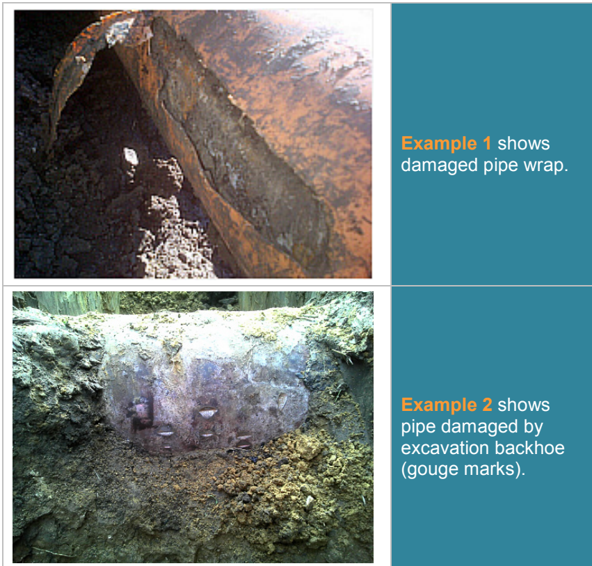
Figure 2. Example of Abnormal Operating Condition (AOC)
