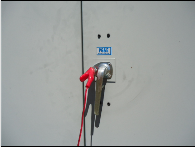
Figure 7. Conductive (Electric Panel)
