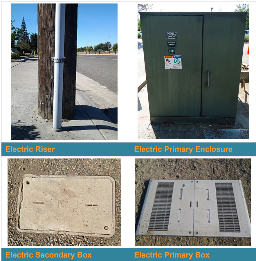
Figure 2. Examples of Energized Facilities
