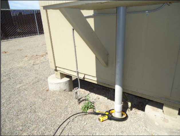
Figure 11. Inductive Clamp (Electric Service Riser)
