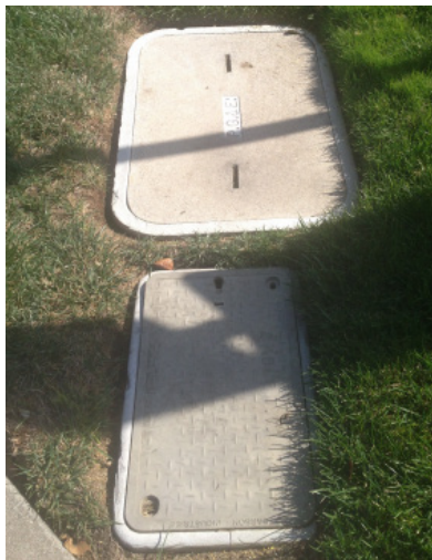
Top: Subsurface Secondary Enclosure (No QEW required for entry)
