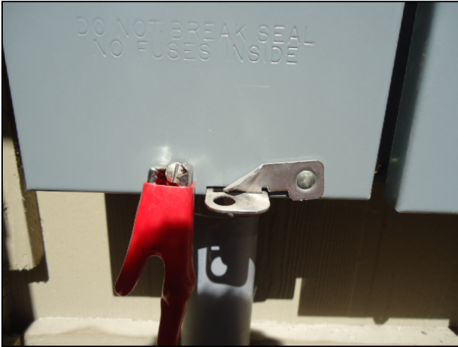
Figure 9. Conductive (Electric Service Meter)
