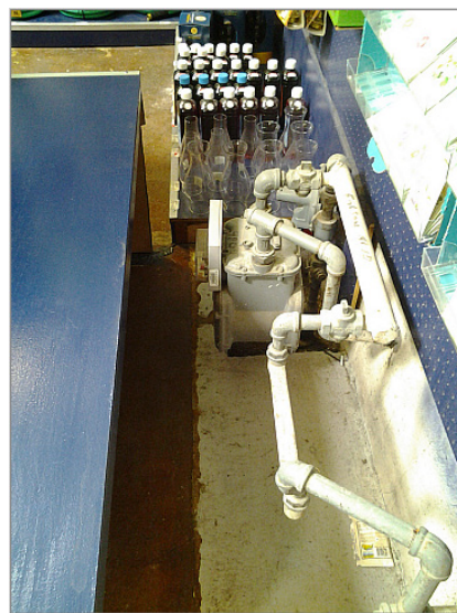
Example 2: Gas meter is inside a building without proper ventilation.
