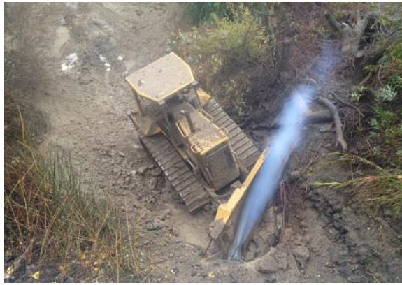
Figure 1. Excavation without a Standby
