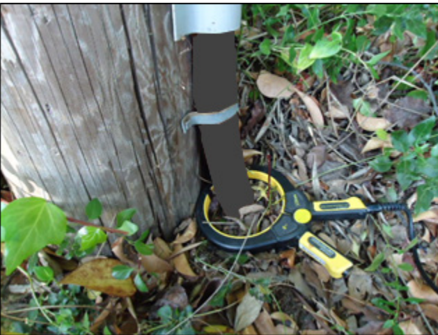
Figure 12. Inductive Clamp (Electric Riser at Pole)
