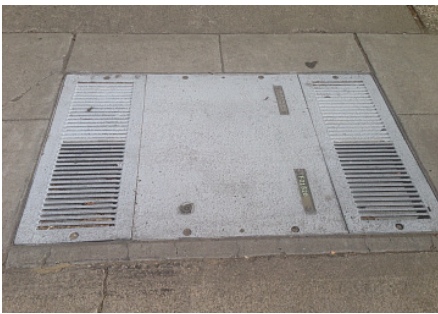
Subsurface Transformer Enclosure (QEW required for entry)
