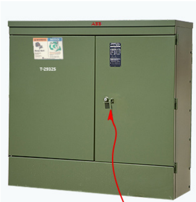
Figure 8. Conductive (Pad-mounted Transformer)
